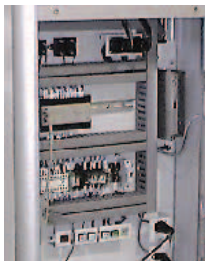
Internal control panel
