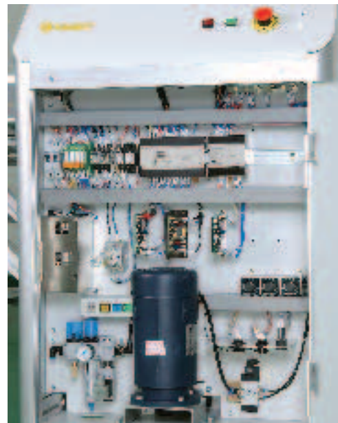
Internal control panel
